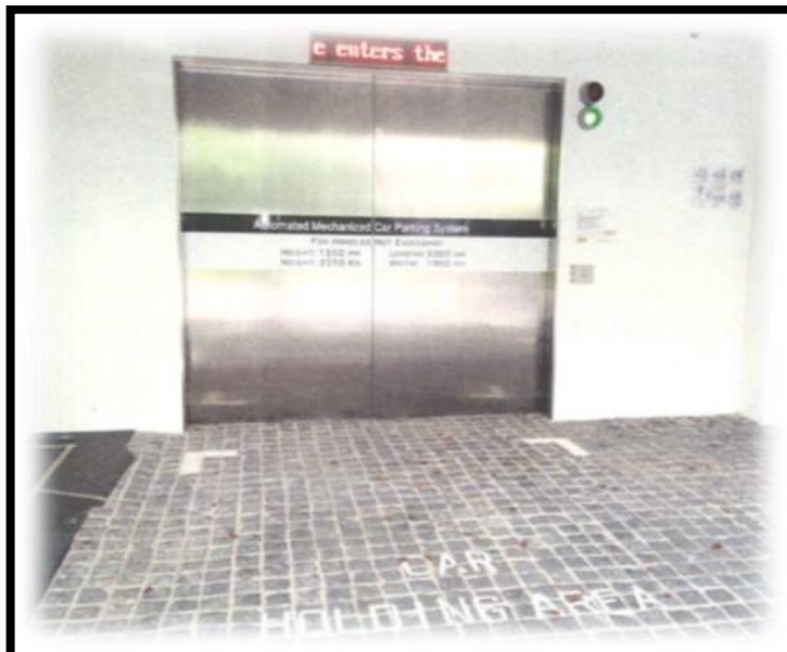
Fig 3.1a Entry point of fully-automated system
