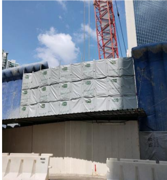
Picture 2 – Silent Up Noise Barrier implemented by Penta Ocean Construction Co Ltd – Bachy Soletanche Singapore Pte Ltd Joint Venture
