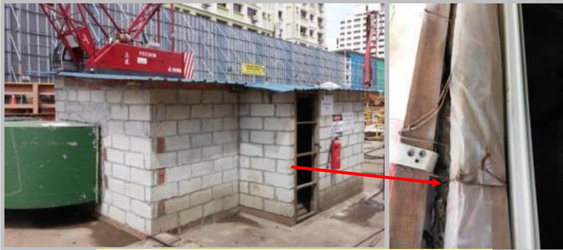
Use of celcon block walls with built-in rockwool to house noisy ventilation fan
