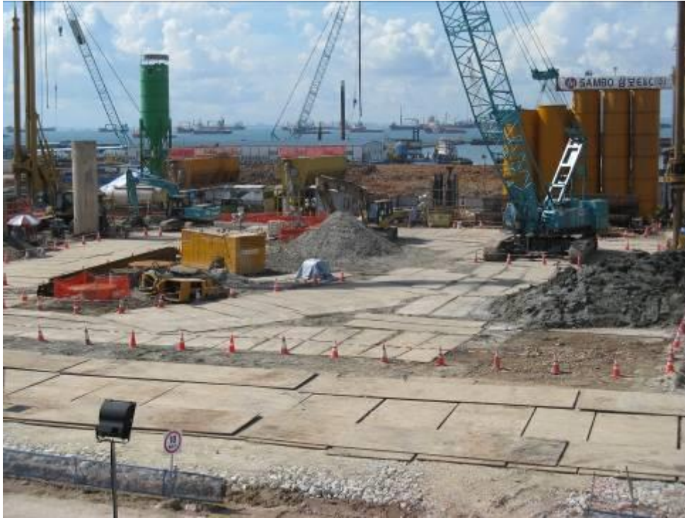
Crane access lined with closely decked steel plates to ensure stability of crane
