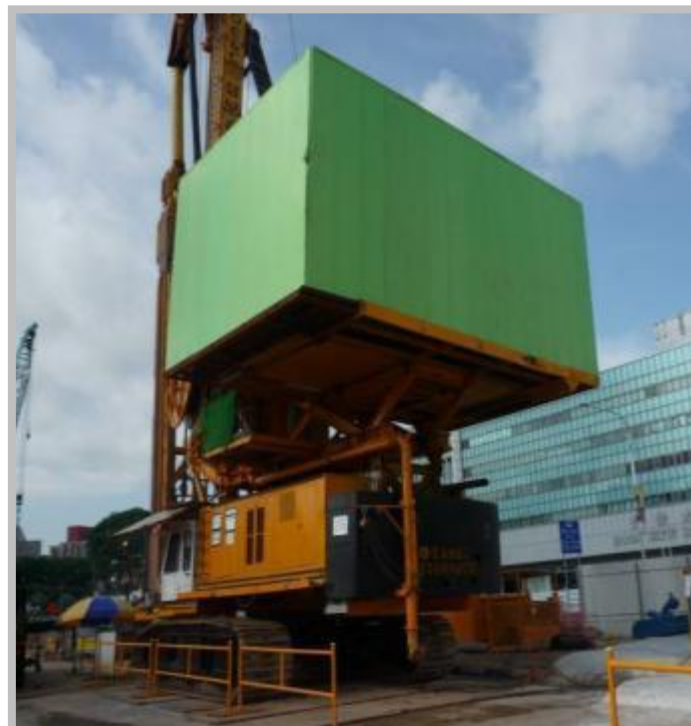
Use of noise enclosures for noisy machineries (For e.g. power-pack generator)
