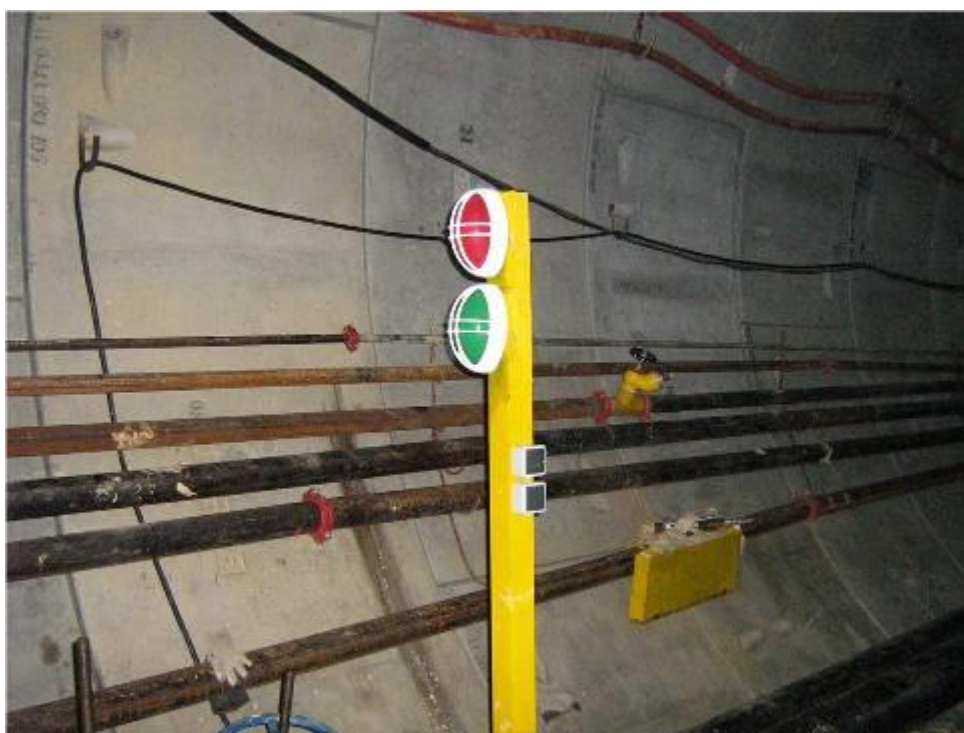
Red and Green signal light to regulate locomotive movement in the tunnel
