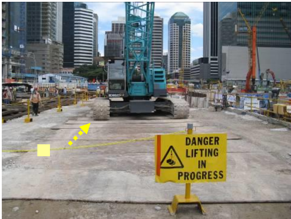
Crane access lined with closely decked steel plates to ensure stability of crane
