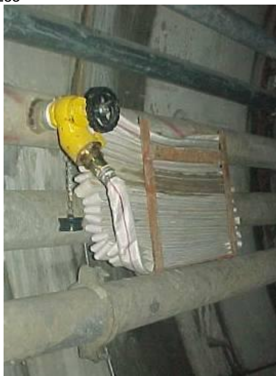
Fire hose reel provided at regular interval along tunnel for fire fighting purpose
