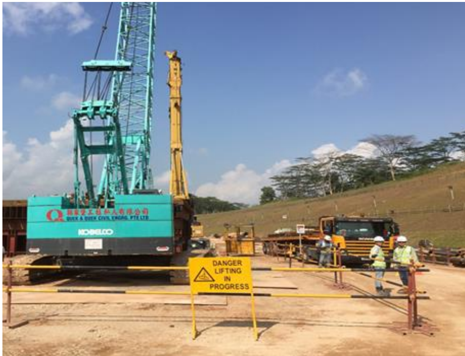
Lifting activity is cordoned off and warning signage is placed to warn personnel against entering the area
