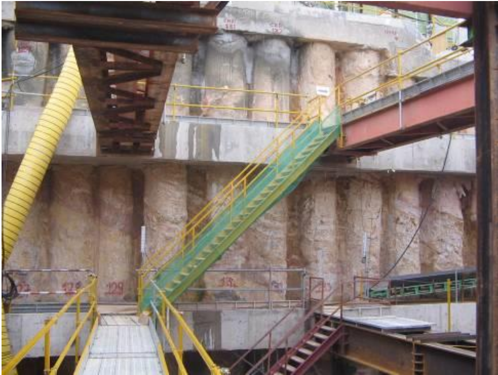
Steel staircase with unobstructed headroom and netting wrapped around handrail and underneath of steps to prevent loose material from falling through
