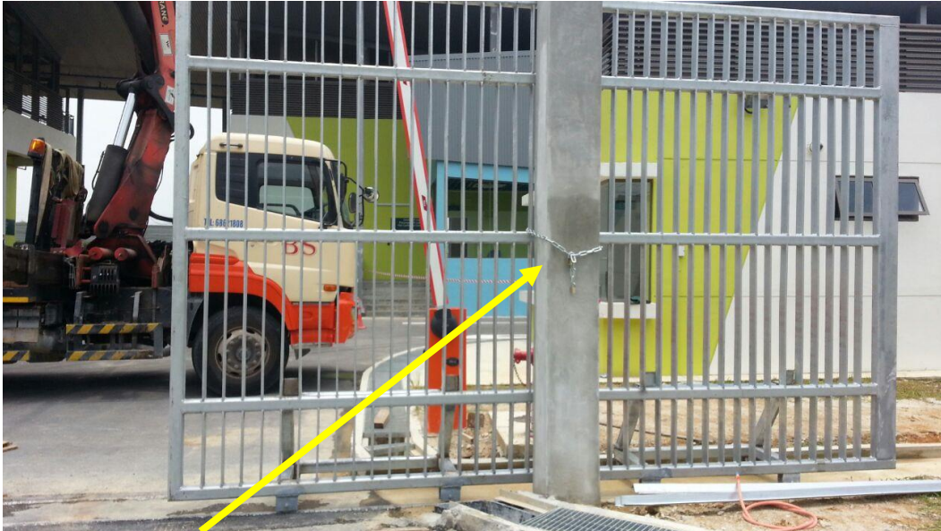
Sliding gate restrained from movement by securing to gate post.
