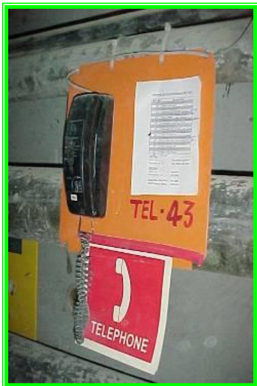
Telephone provided at regular interval along tunnel to notify of any emergency
