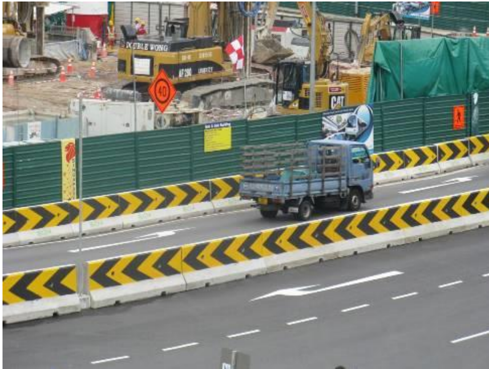
Concrete barriers use to protect workers against the possibility of vehicles crashing into site boundary
