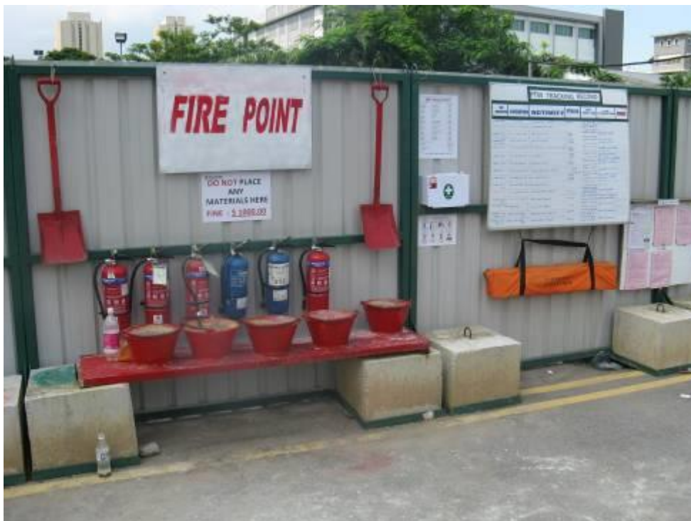
Fire fighting and first aid equipment readily available at strategic locations
