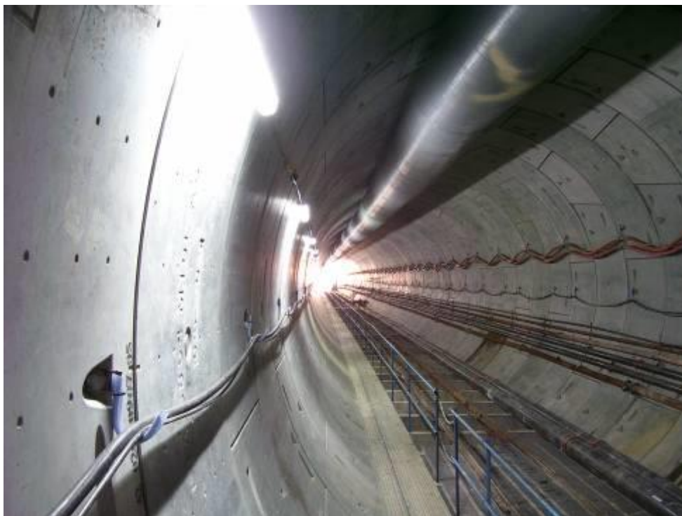
Continuous walkway with guardrail provided along the tunnel
