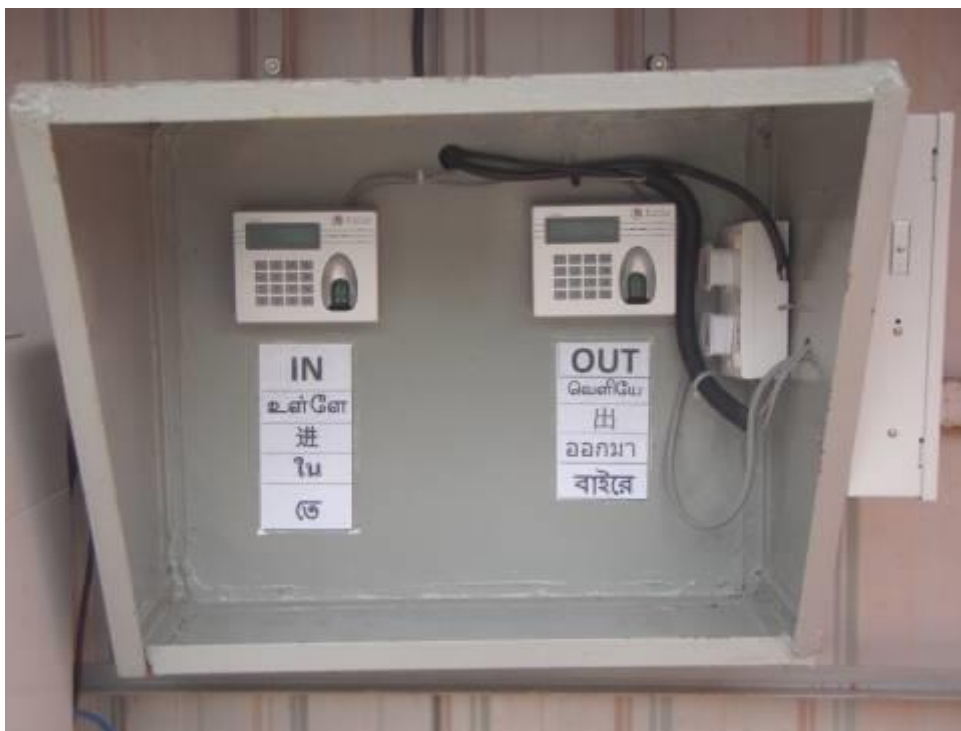
Access control to Tunnel using finger print. This method eliminate the problem of forgetting to bring or loss of identification tags
