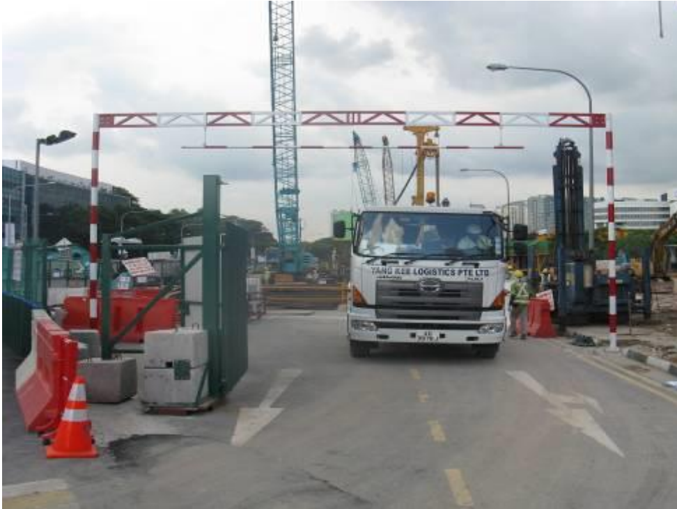
Height Limit Gantry installed at site entrance / exit to ensure the total height of the vehicle does not exceed 4.5m
