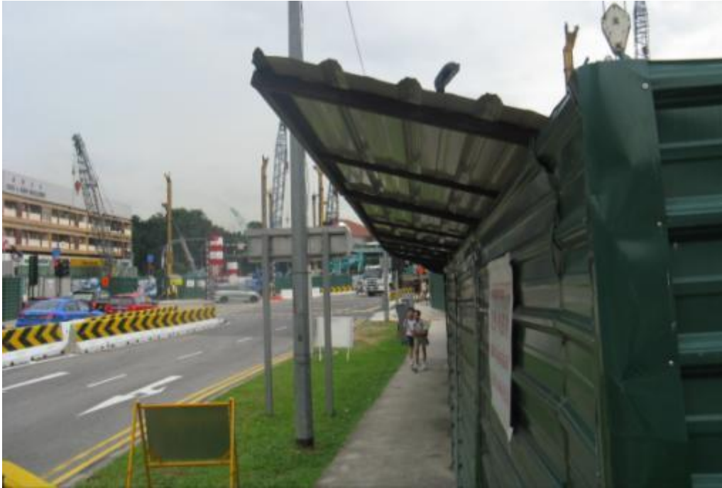
Overhead shelter provided when work is carried out near hoarding to protect the public from any falling objects
