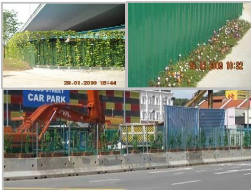
Use of 'green' hoardings to beautify the site and to reduce the impact from traffic carbon emissions
