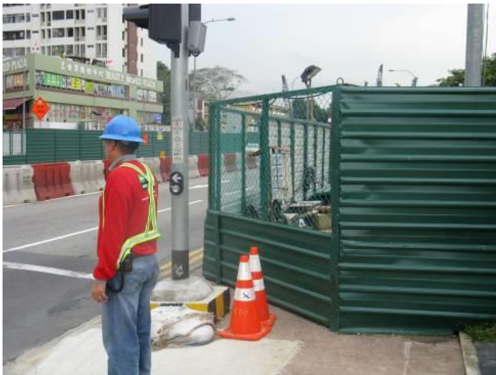
“See through fencing” allows pedestrian to check and ensure vehicles has stopped before crossing at traffic junction
