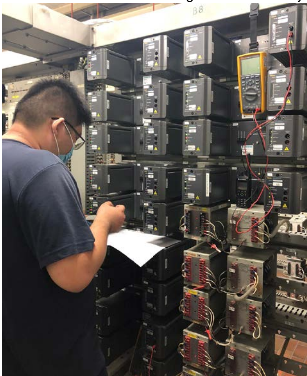
Photo 2: Testing works for the new track circuit system to ensure stability of the system.
