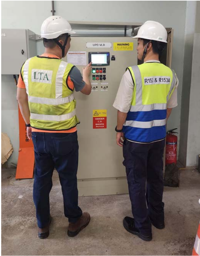
Photo 3: The new power supply system features new Voltage Limiting Devices, which isolates power faults to prevent line-wide disruptions.
