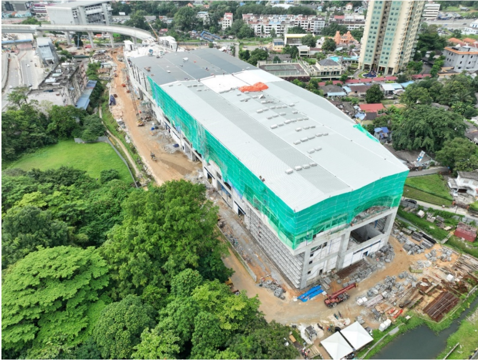
RTS Link Maintenance Depot
