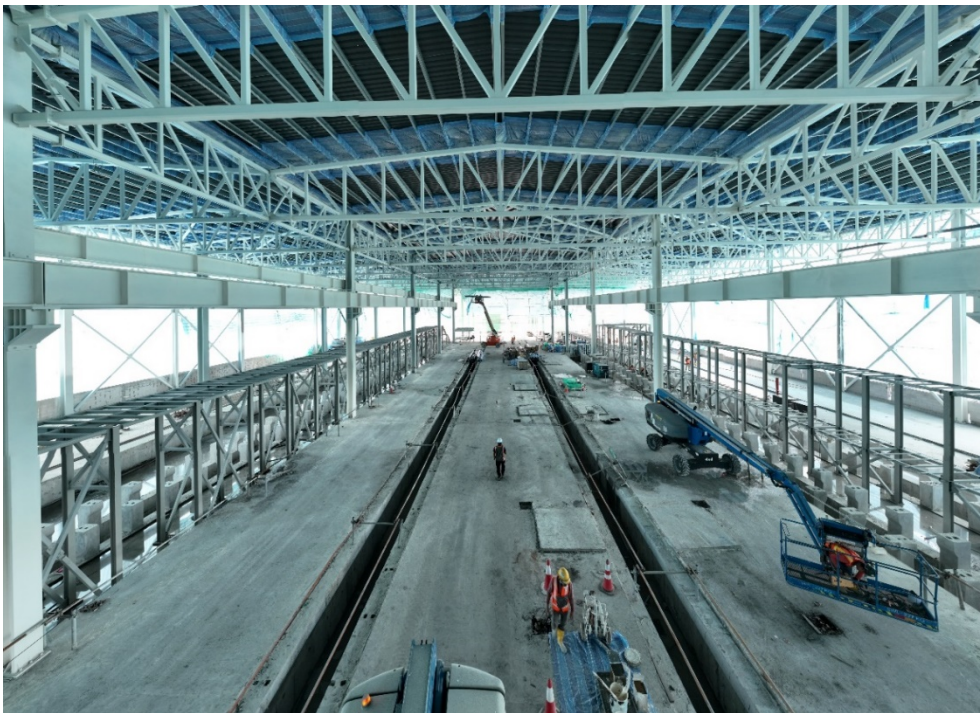
RTS Link Maintenance Depot
